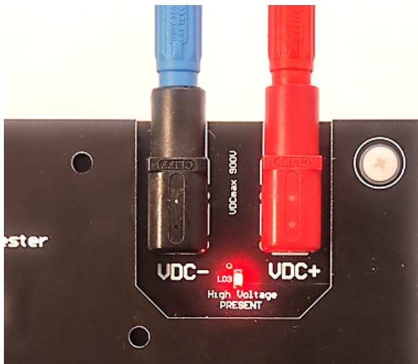
Figure 8. High Voltage Present
